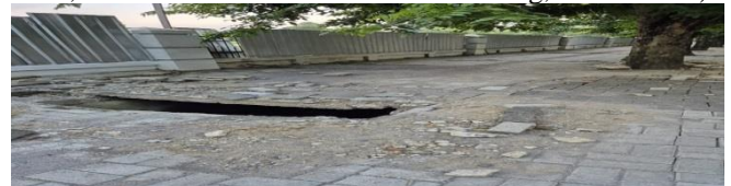
(a) Damaged pedestrian path
